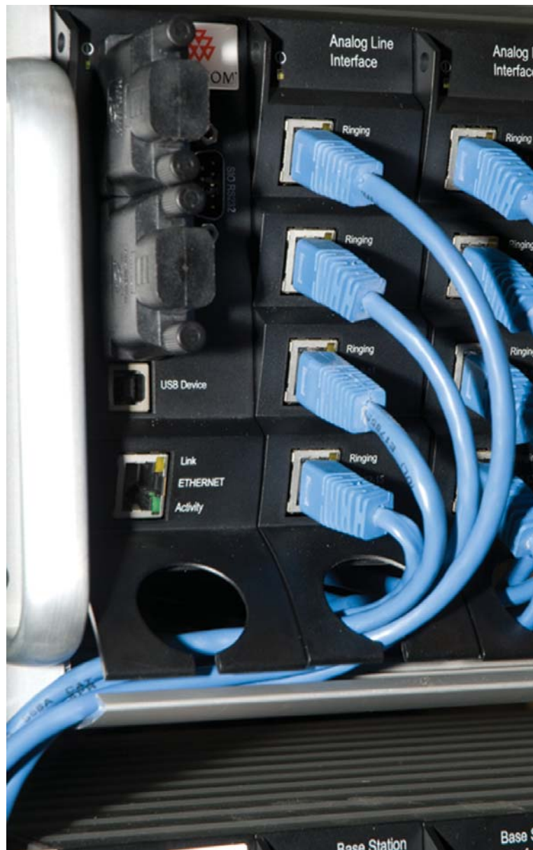
Figure 11 Harnessing cables to the side and out.
